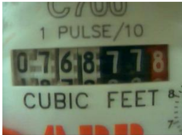
Figure 16 Original utility meter image #1
