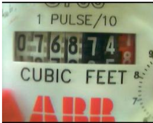
Figure 35 Example of failed utility meter reading
