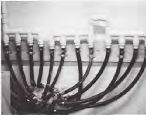
Pipes for underground circulation of water enter through cellar wall.
