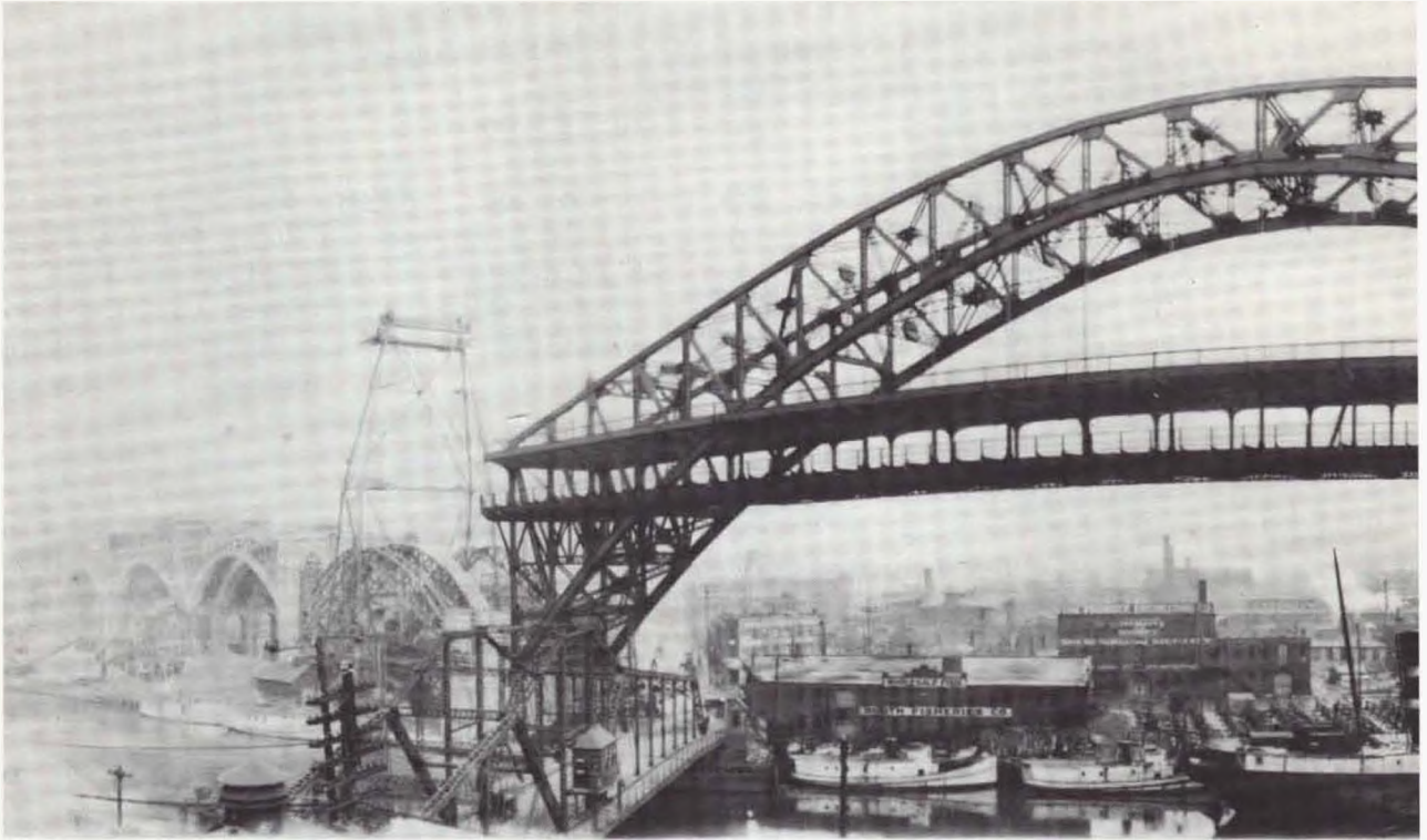
1. Detroit-Superior High Level Bridge Under Construction, (1916); Left foreground, Center Street Bridge, (1901); Right foreground, Cleveland Milling Company (Fairchild), wheat being unloaded into elevator.
