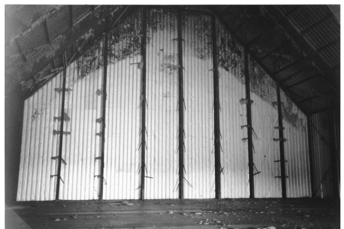
Fig. 4. Column flange braces torn away at end wall
