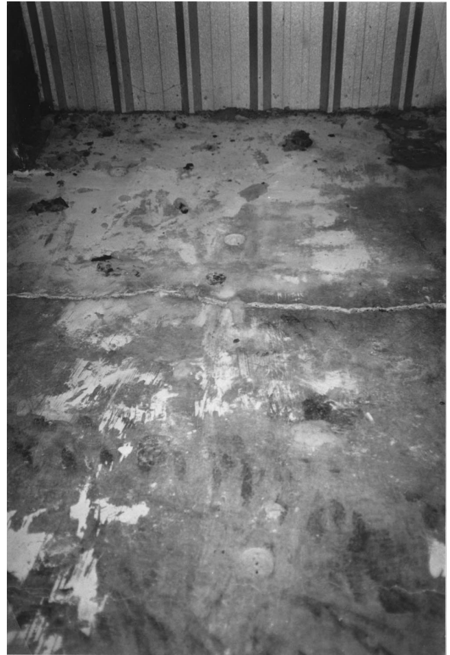
Fig. 7. Cracking near end wall, warehouse 2
