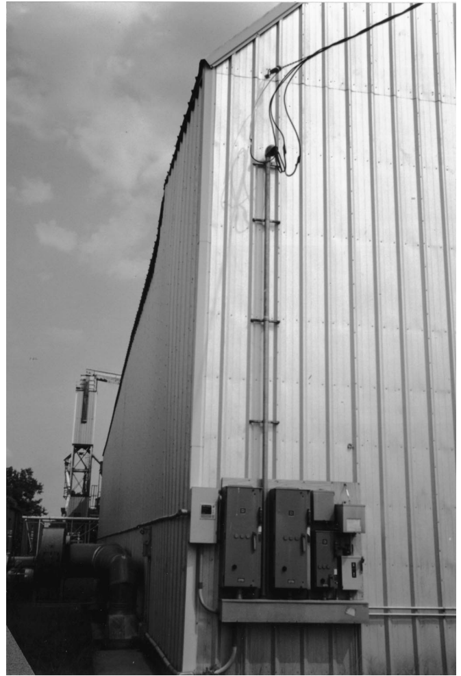
Fig. 3. Damage at eave line
