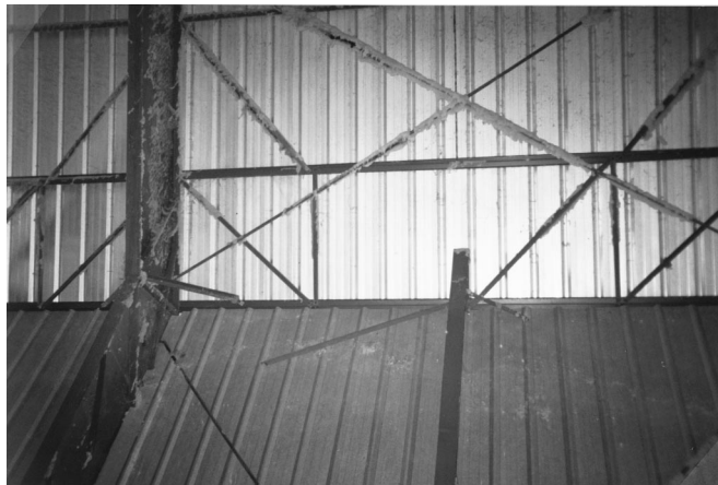
Fig. 6. Interior column brace torn, warehouse 2
