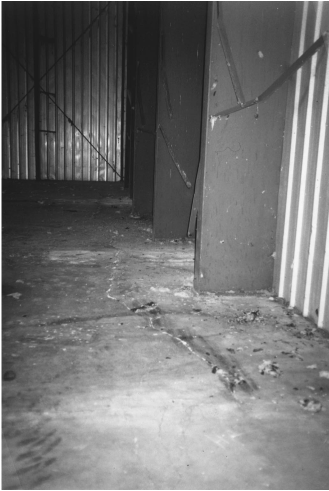
Fig. 5. Cracking near side wall columns
