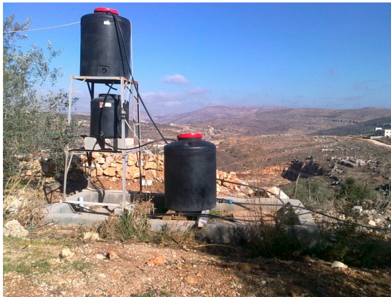
Figure 1. Onsite grey water treatment plant, Duara Al Qare'-Ramallah.
