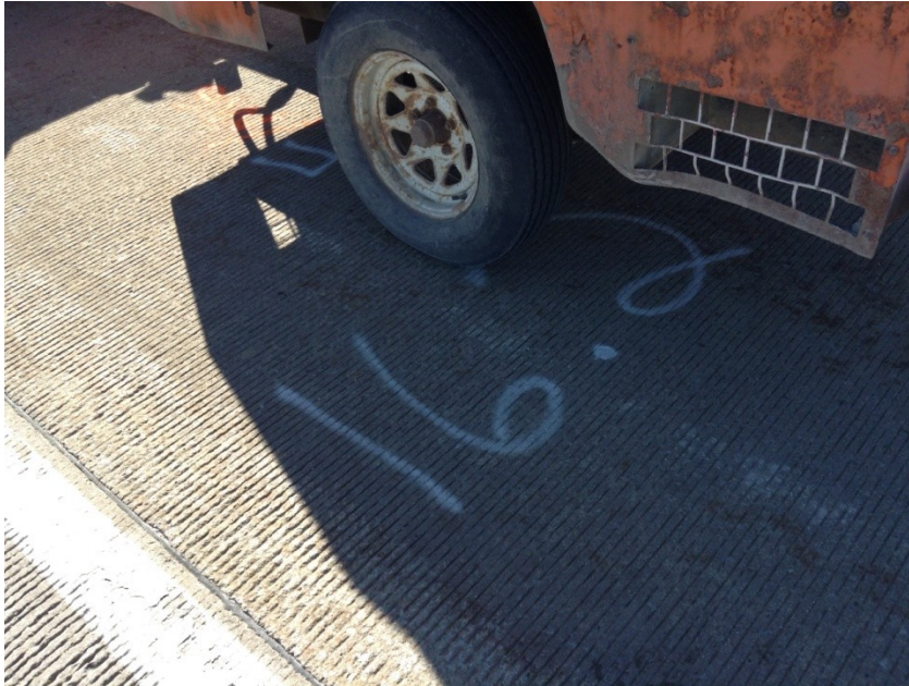
Figure 15: Mile marker location for patches #9 and #10.
