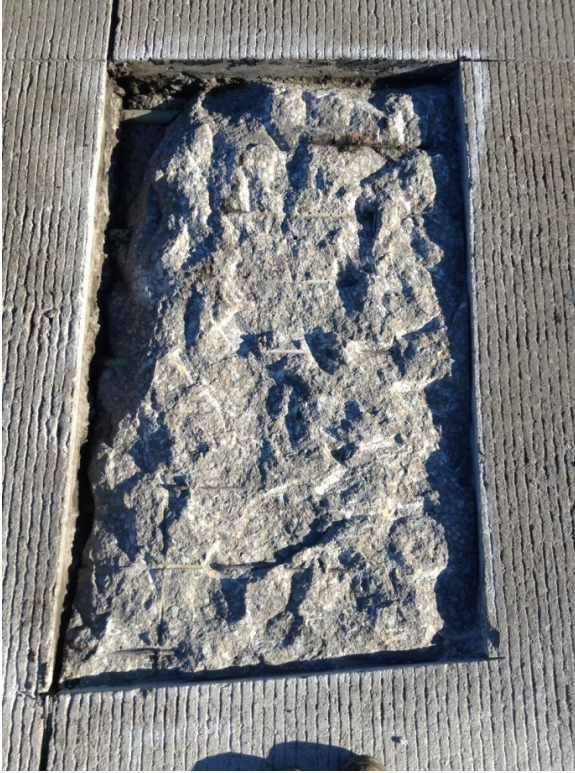
Figure 20: Patch #5, placed at an expansion joint, visibly damp at upper-left corner.
