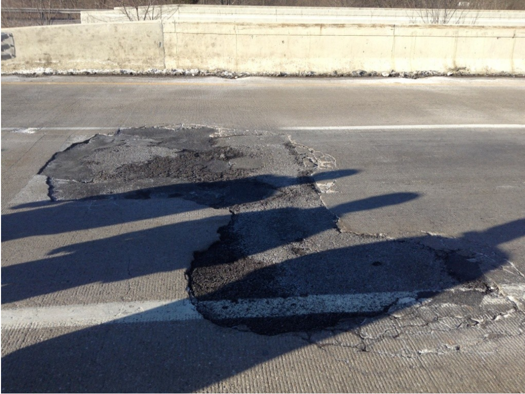
Figure 6: Previous patch deterioration, at location of patches #2 and #3.
