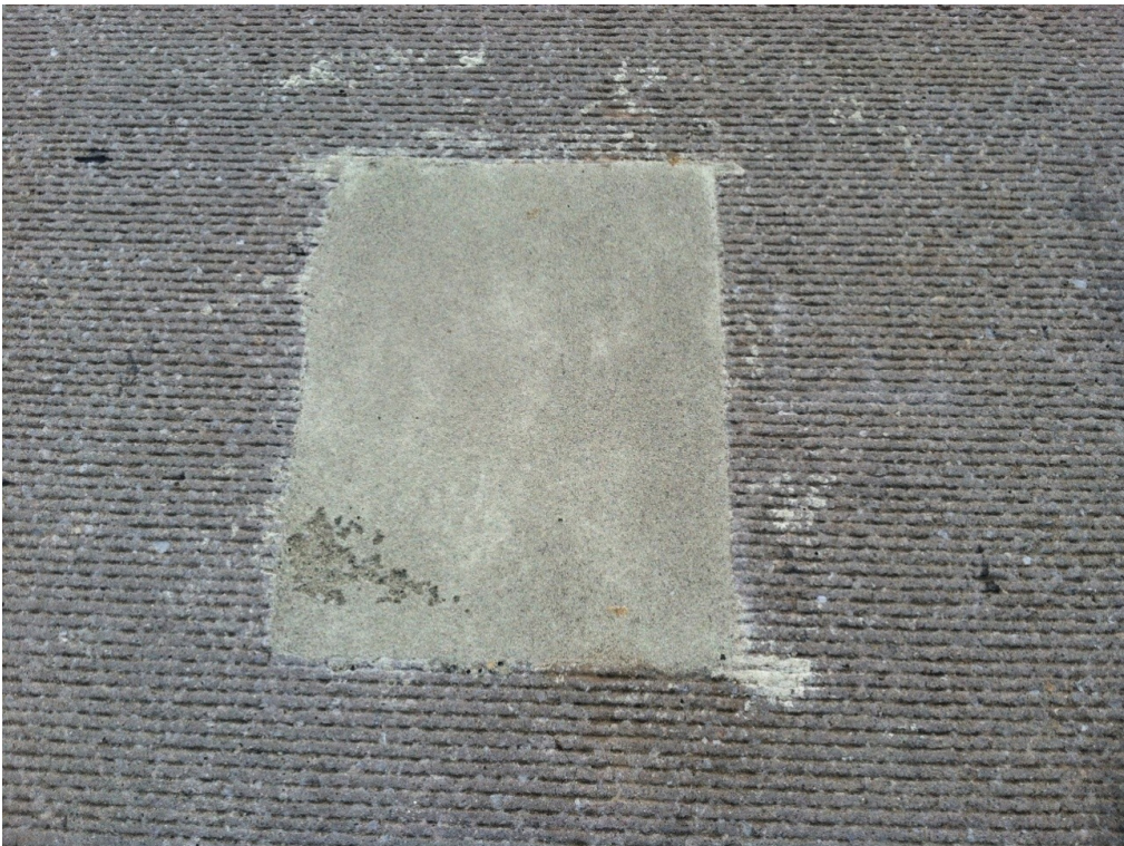
Figure 31: Patch #8, constructed with Flex Set, showing slight surface spalling on the bottom left of the patch.
