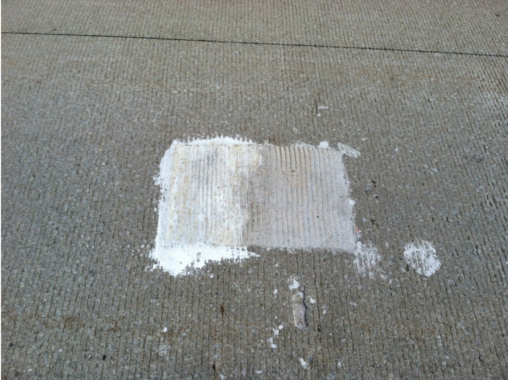
Figure 35: Patch #6, containing MG Krete, with the improper mixture proportioning still visible.
