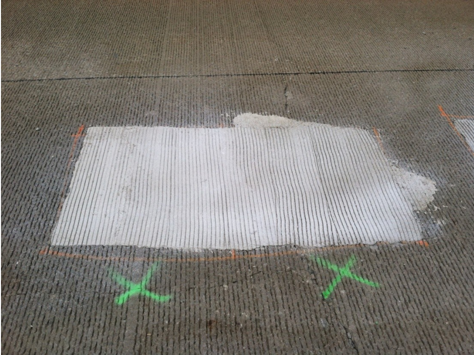
Figure 29: Patch #64, containing FastSet DOT Mix, with a crack running through the concrete slab and under the patch.
