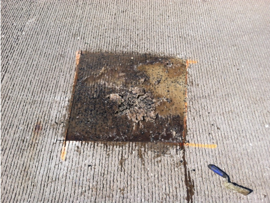
Figure 25: Patch #21, containing SR-2000, in which the entire patch did not set. The patch was cleared and refilled after the patch did not set over the course of 5 hours.
