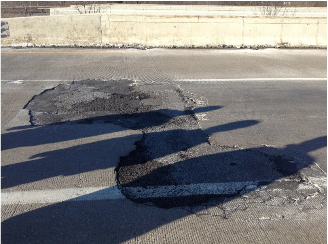
Figure 3: Failing patch on bridge deck, before installation of new patches.
