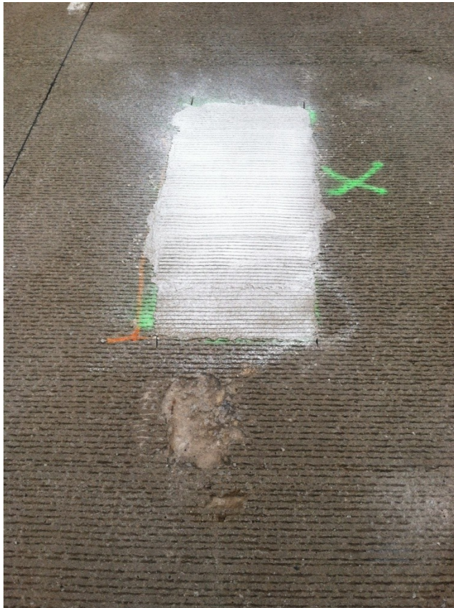
Figure 28: Patch #68, containing FastSet DOT Mix, with a pothole in front of it. Delamination was detected between the patch and the pothole after installation.
