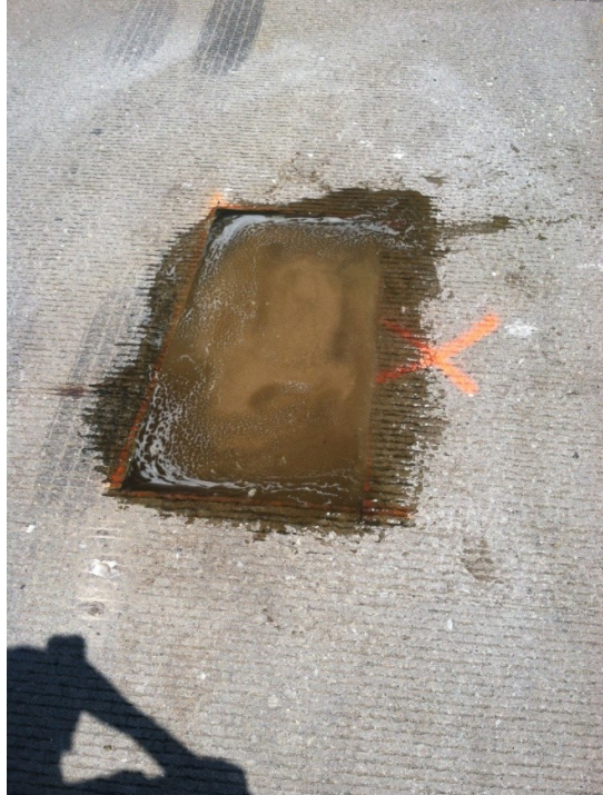
Figure 24: Patch #26, containing SR-2000, bleeding liquid.
