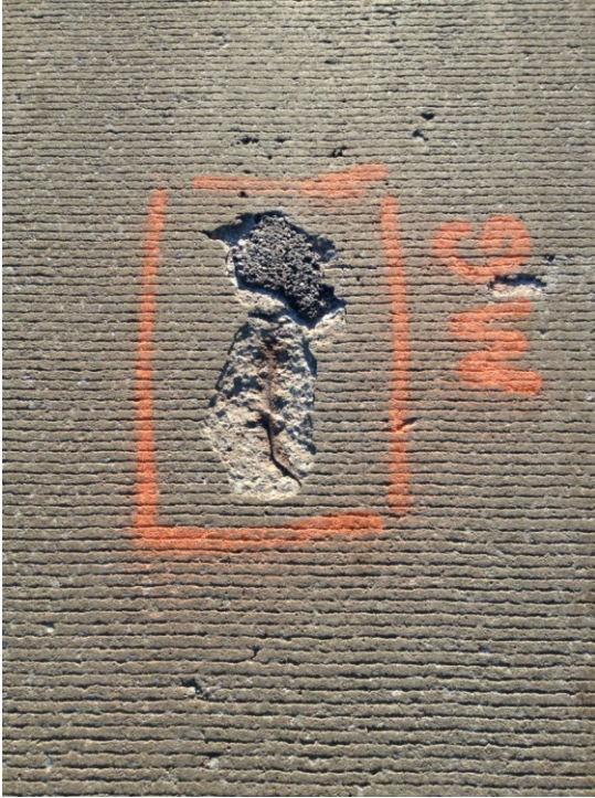
Figure 7: Spalling, at location of patch #6.
