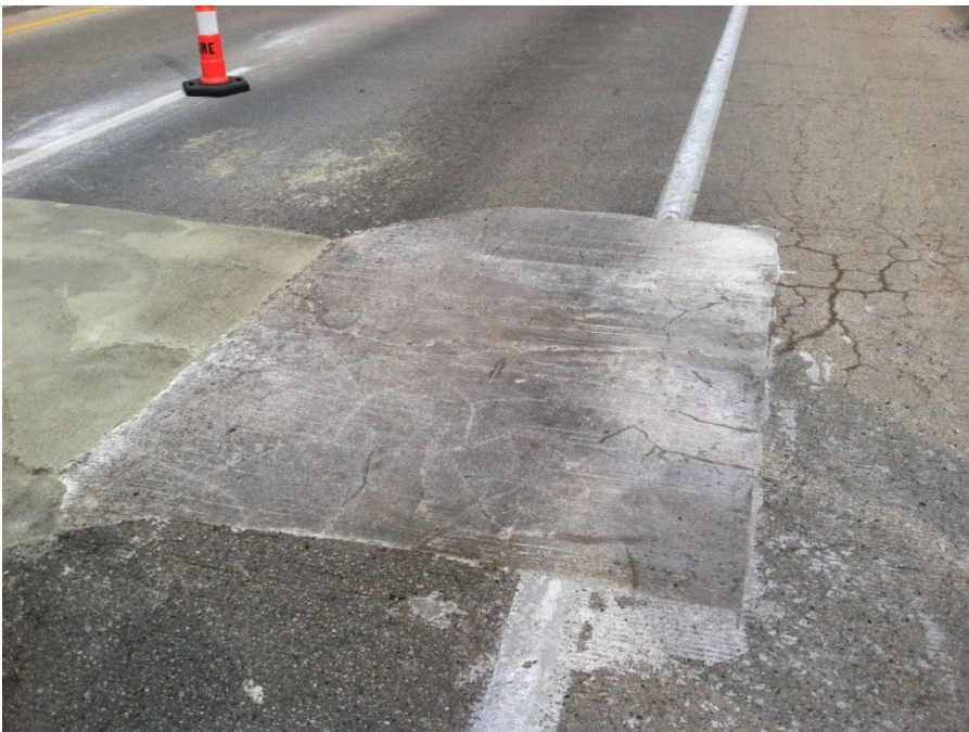
Figure 33: Patch #1, containing MG Krete, and showing cracking 2.5 months after installation.
