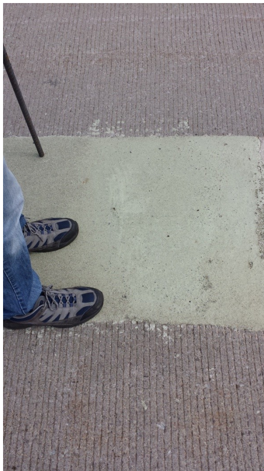
Figure 32: Performing the rebar test on patch #11, containing Flex Set, with the rebar placed over the area that failed the rebar test.
