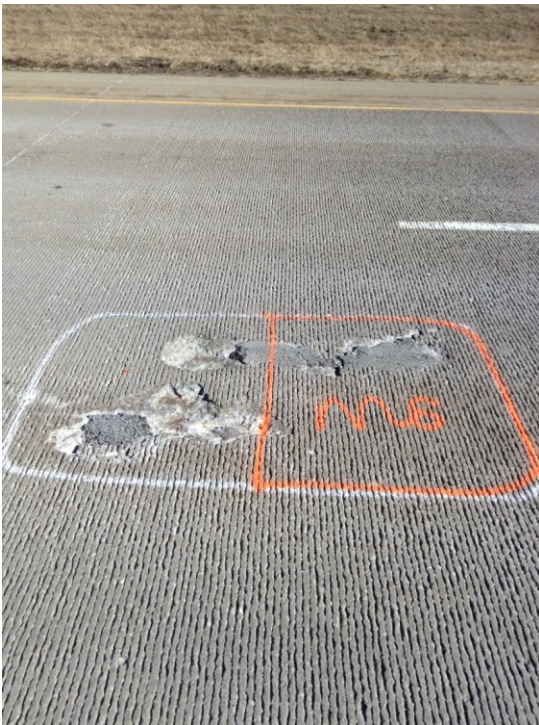
Figure 8: Spalling and potholes at location of patches #9 and #10.
