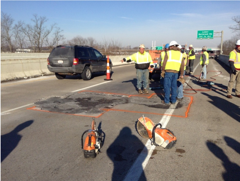
Figure 9: Outlining the proposed patch areas with spray paint.
