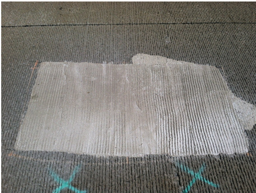
Figure 36: Patch #64, consisting of FastSet DOT Mix, with a small crack through the patch.
