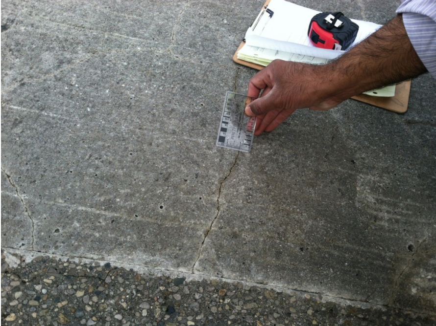
Figure 34: Patch #1, containing MG Krete, and showing a crack that is approximately 1/32 inches (0.79 mm) wide, 2.5 months after installation.
