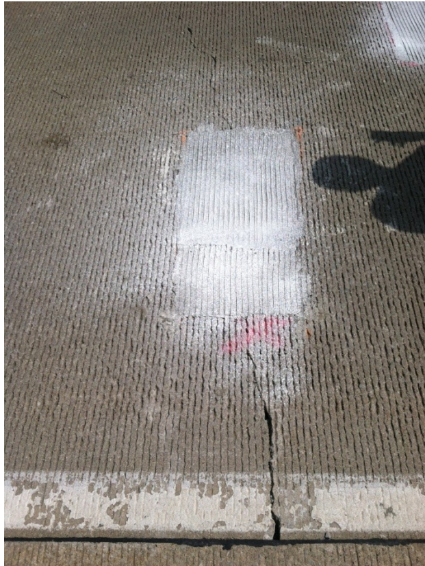
Figure 30: Patch #76, containing RepCon 928, with a large slab crack running through the middle of the patch.
