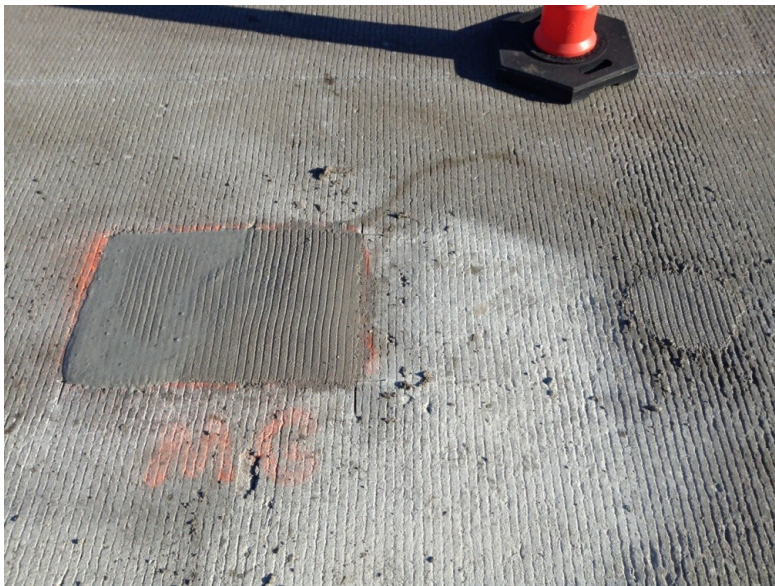
Figure 23: Patch #6, constructed with MG Krete, showing bleeding in the left half of the patch due to improper mixture proportions.
