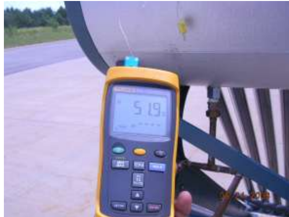
Figure 16: Temperature Measurements. Courtesy: [HMI Industries]
