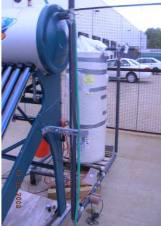
Figure 19: Piping from Solar water heater to HWT. Courtesy: [ HMI Industries]
