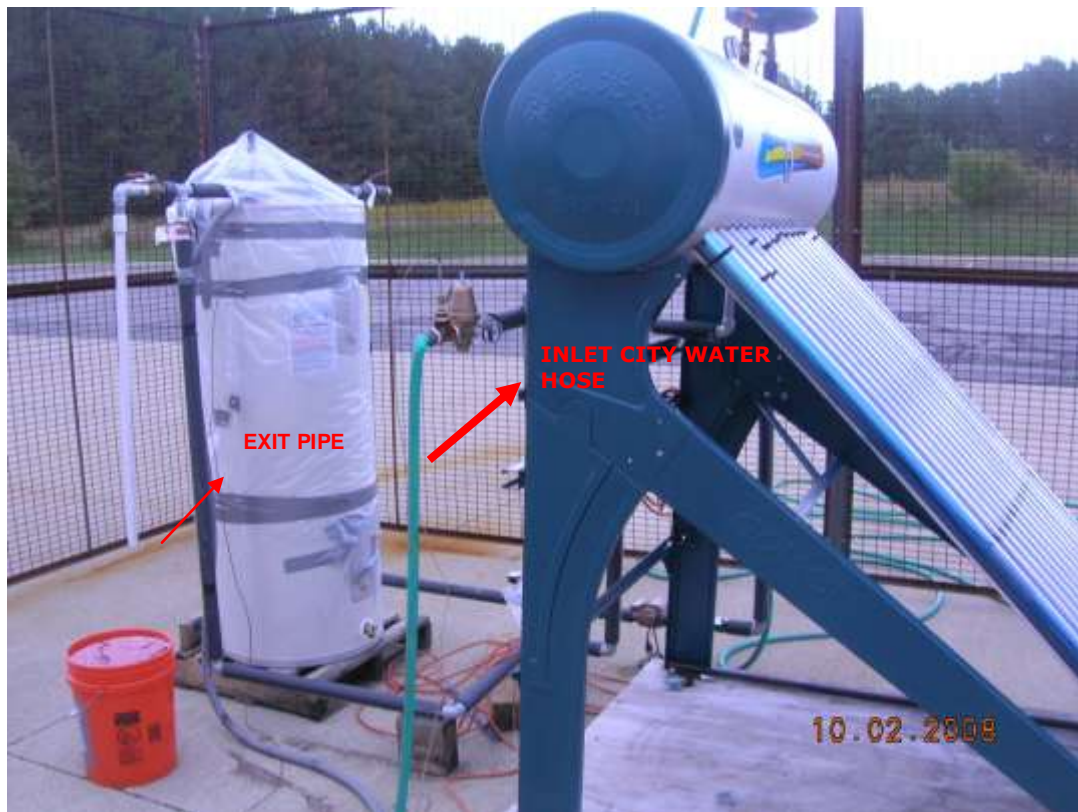
Figure 22: Solar Water Heater connected in series with the Hot Water Tank. Courtesy: [HMI Industries]
