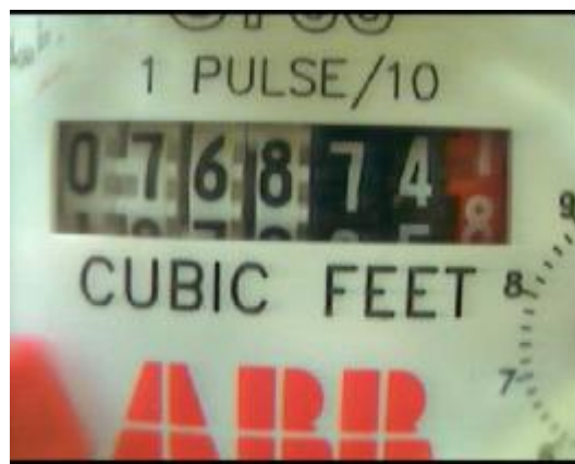
Figure 35 Example of failed utility meter reading
