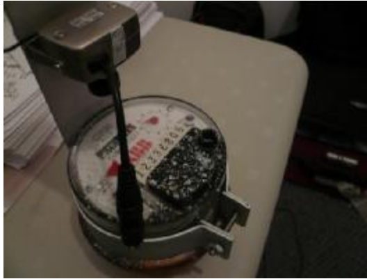
Figure 22 The wireless camera and gas meter
