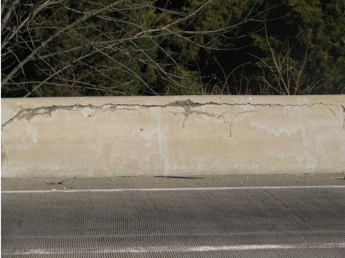
Figure 27: Bridge Number HAM-74-1116L Cracking (Photo Provided by Brandon Collett, PE)
