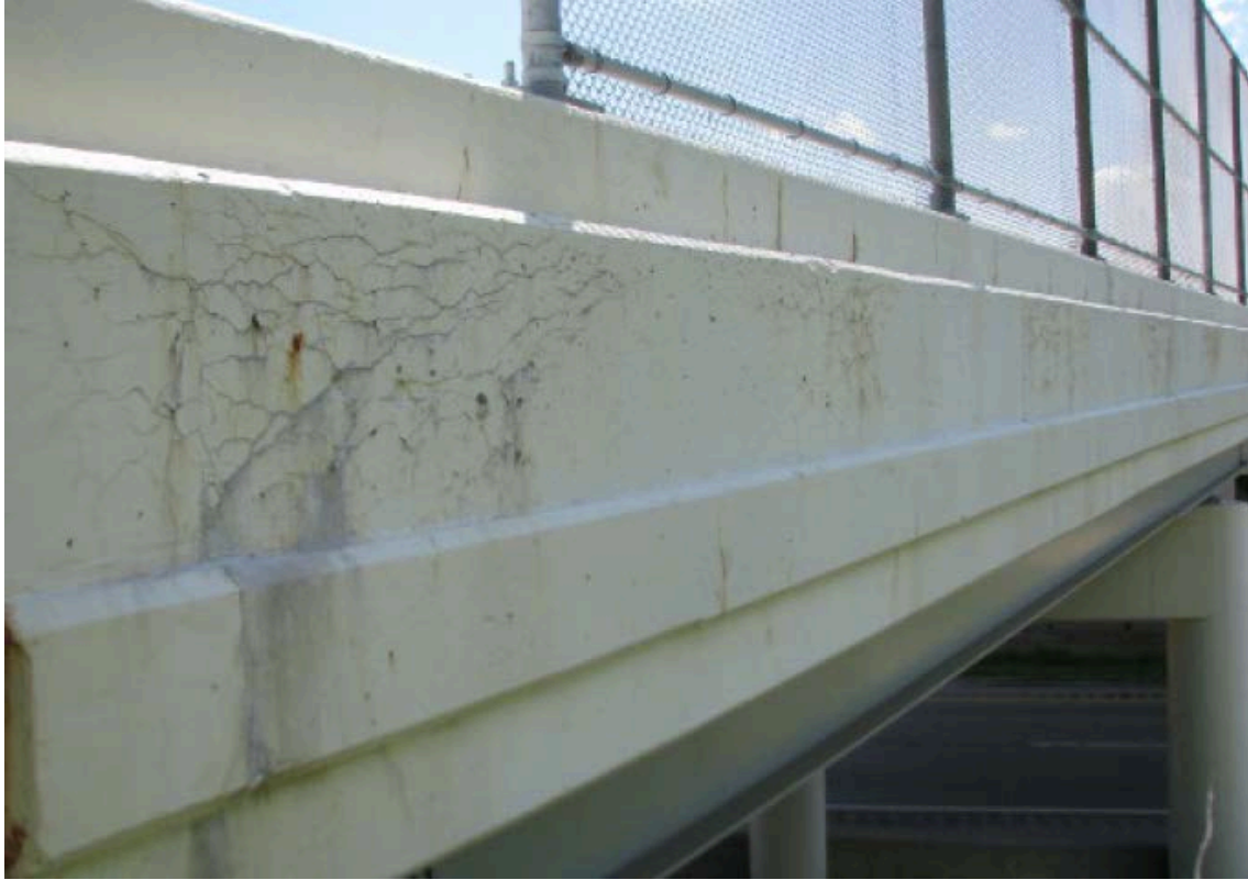
Figure 30: Bridge Number GRE-380-0671 Cracking (Photo Provided by Brandon Collett, PE)
