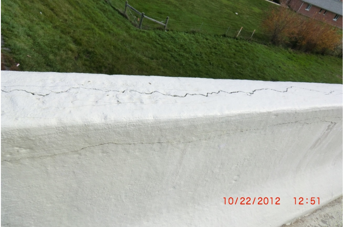
Figure 23: Bridge Number ALL-75-1836 Cracking (Photo Provided by Rod Maas)
