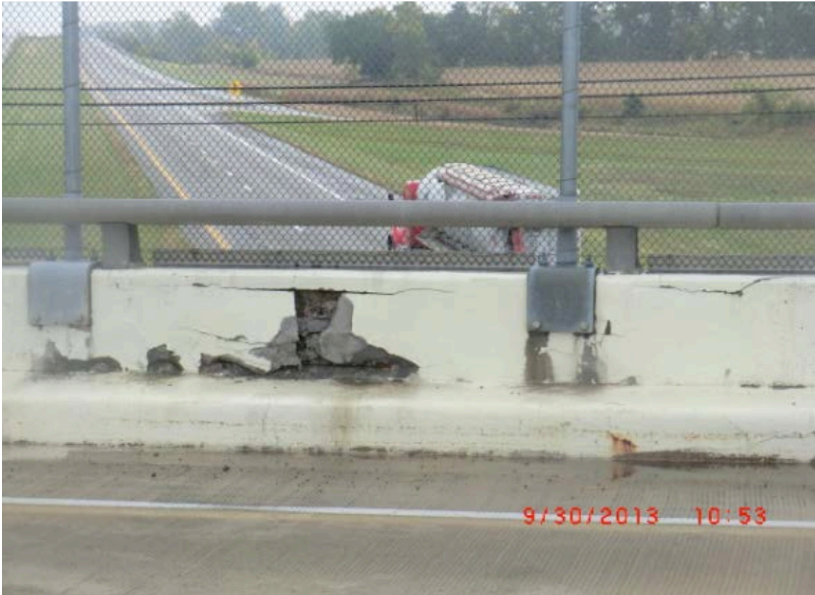
Figure 25: Bridge Number ALL-65-1322 Cracking (Photo Provided by Steve Reichenbach)
