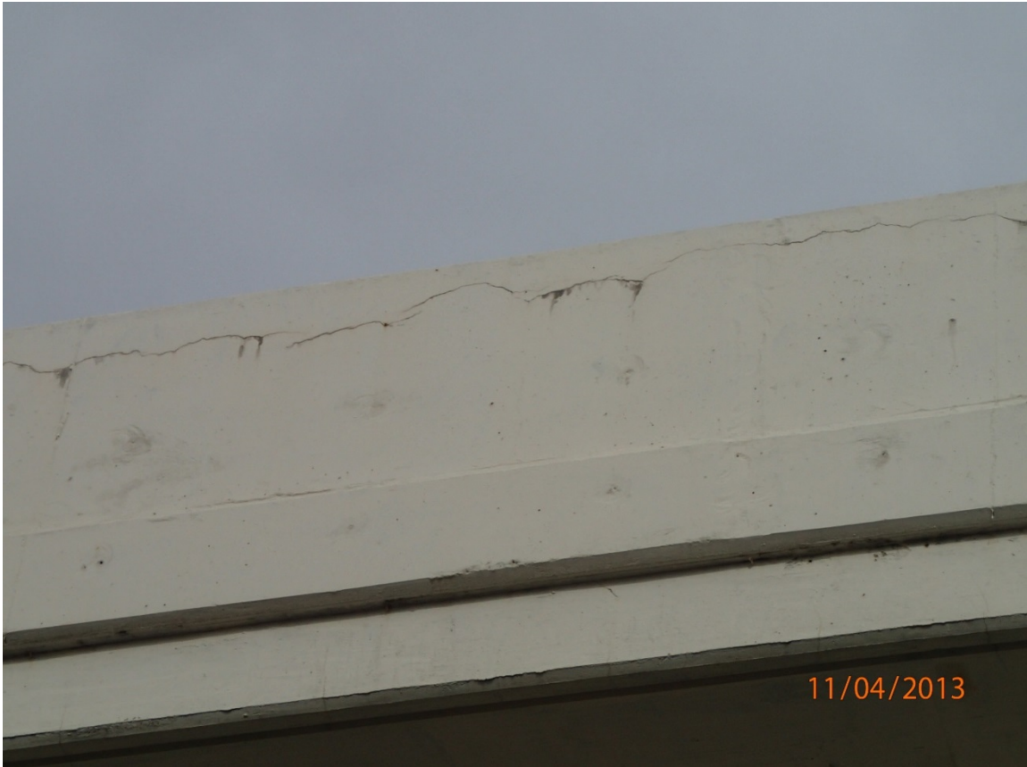
Figure 24: Bridge Number ALL-696-0086 Cracking (Photo Provided by Rod Maas)
