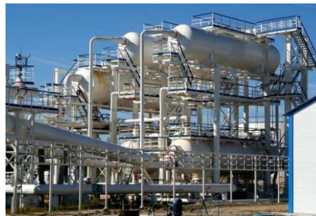
Photo: Oil Separator Complex by Yukon White Light
